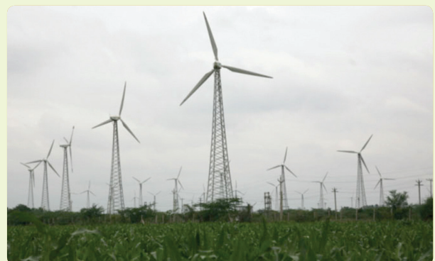
Clean Energy of 12 MW capacity generated by JKM Wind Farm at Coimbatore - a step towards achievement of zero carbon footprint.
